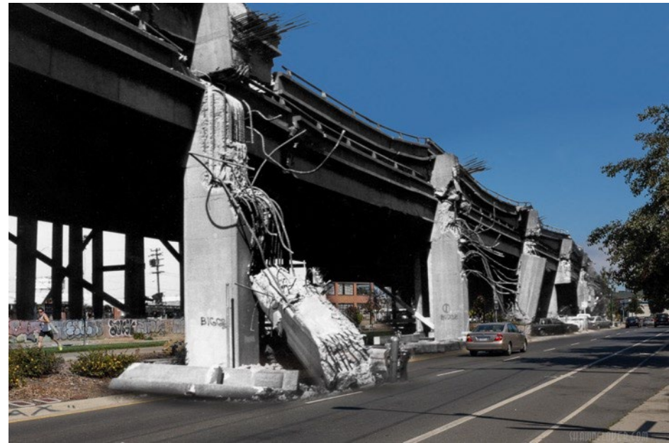
Embarcadero Freeway 1989 Loma Prieta earthquake damage!
