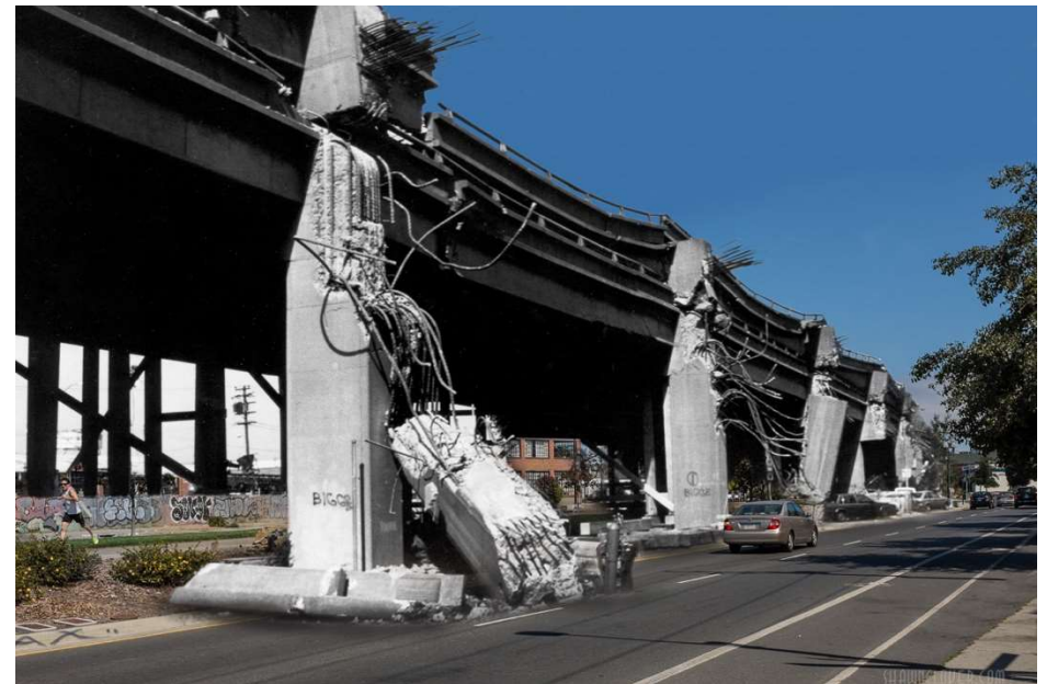
Embarcadero Freeway 1989 Loma Prieta earthquake damage!
